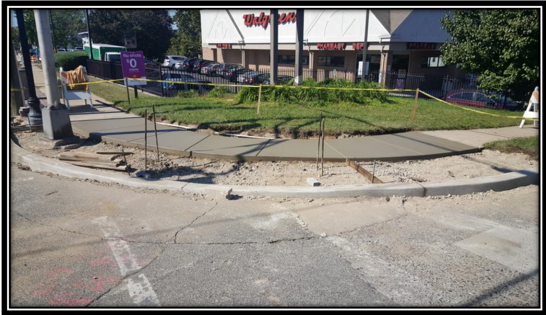
Figure: 2 – Installation of concrete sidewalk at northwest corner of the intersection with 47th Street along the westbound lane
