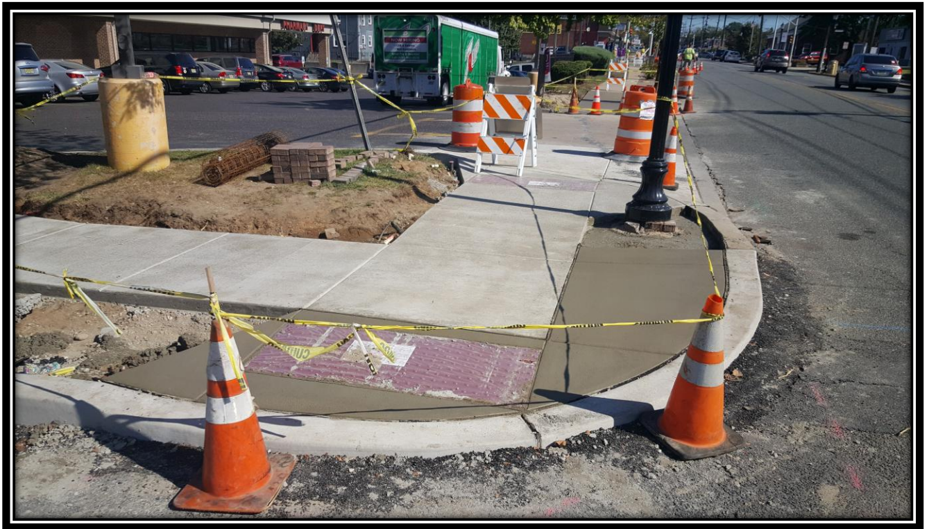
Figure: 1 – Installation of a concrete ADA ramp at the northeast corner of the intersection with 46 th Street along the westbound lane
