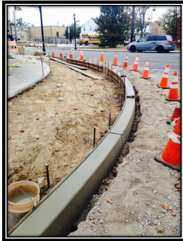
Figure: 3 – Installation of concrete curb at the northeast corner of the intersection with West River Drive along the westbound lane
