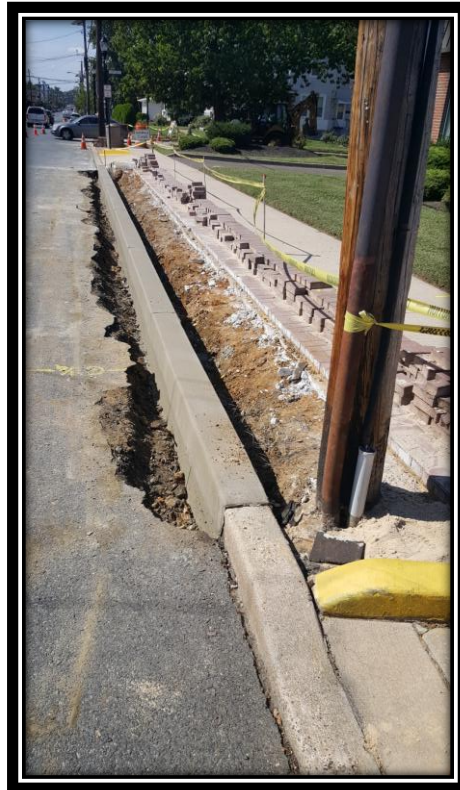
Figure: 1 – Installation of concrete curb along the westbound lane between 43 rd Street and 44 th Street
