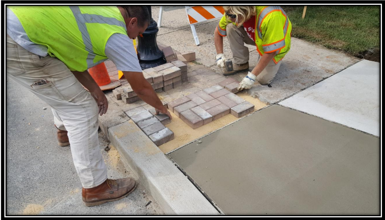
Figure: 2 – Installation of concrete sidewalk and brick pavers along the westbound lane at the intersection with 43 rd Street
