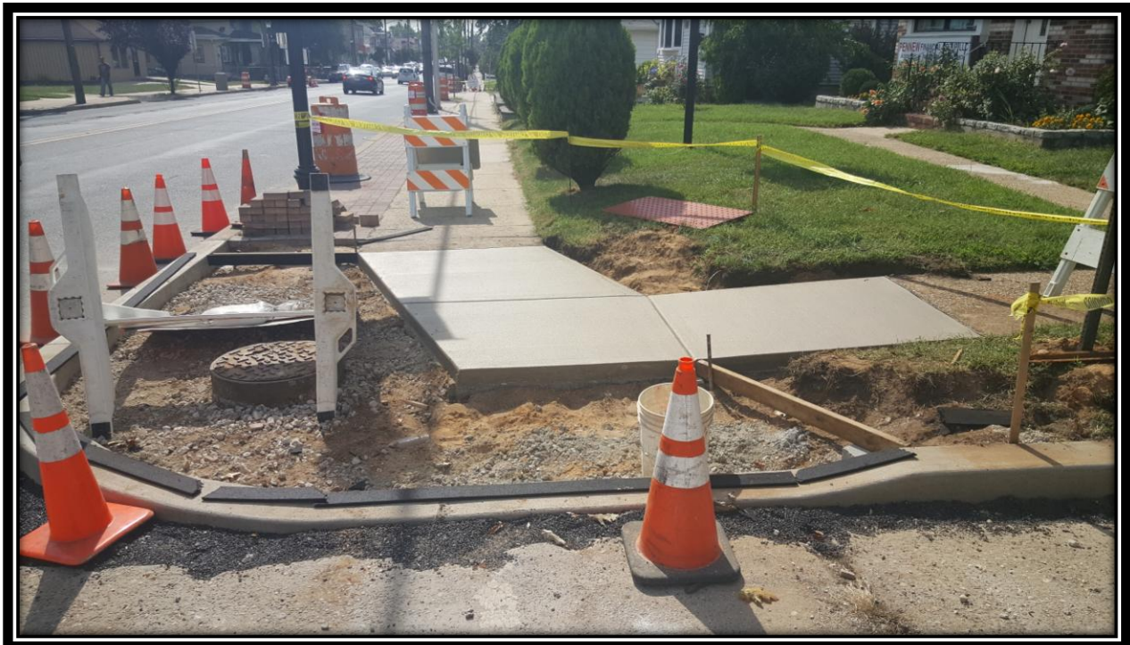
Figure: 3 – Installation of ADA ramp along the westbound lane at intersection with 43 rd Street
